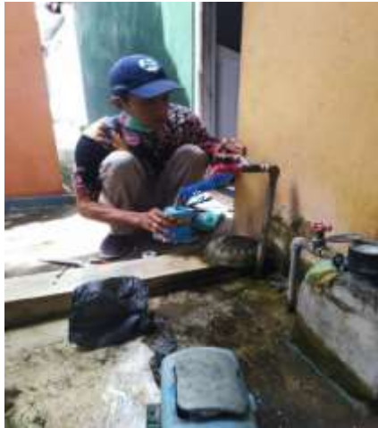
Figure 4. Installation of pressure logger data
