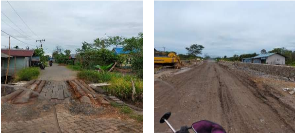
Figure 1. North Ring Road Condition (Road Access to Lok Baintan Floating Market) Severely Damaged Due to Flood
