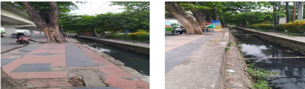
Figure 1. The condition of the pedestrian path on Jalan Andi Pangeran Pettarani
