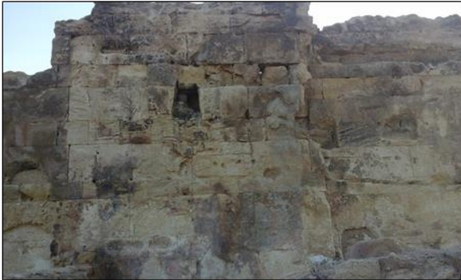
Figure 6. Presence of Salt Efflorescence on the Surface of Limestone
