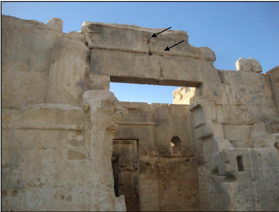
Figure 9. A Fracture in the Threshold Stones on the Main Facade as a Result of the Large Loads and the Weakness of the Salty Limestone (As Arrows Refer)
