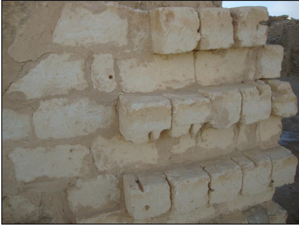
Figure 10. A Loss in the Lower Part of One of the Walls and It has been Completed with New Limestones with Higher Mechanical Properties
