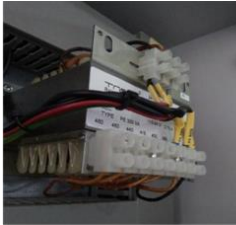
Figure 8. Step Down Transformer in the Control Panel
