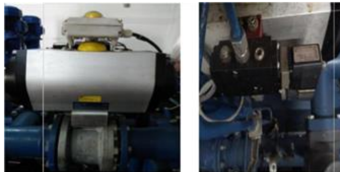
Figure 9. Photo of the Solenoid Valve in the Fuel Feeder of PLTMG Balai Pick Up
