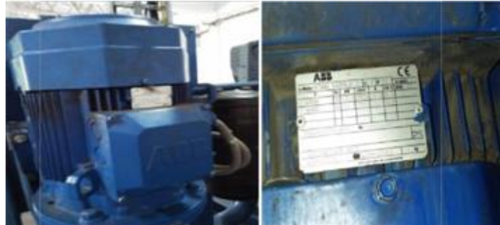
Figure 11. Photo of Pump Motor on Fuel Feeder
