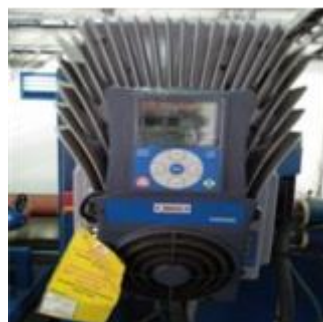
Figure 10. Photo of Frequency Converter in Fuel Feeder PLTMG
