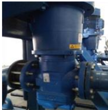
Figure 12. Photo of Fuel Feeder Pump
