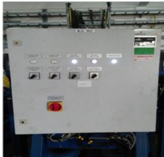
Figure 7. Fuel Feeder Control Panel
