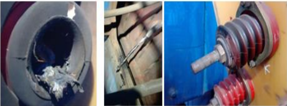
Figure 6. Condition of S-Phase Motor Terminal Burns During Unit Trip
